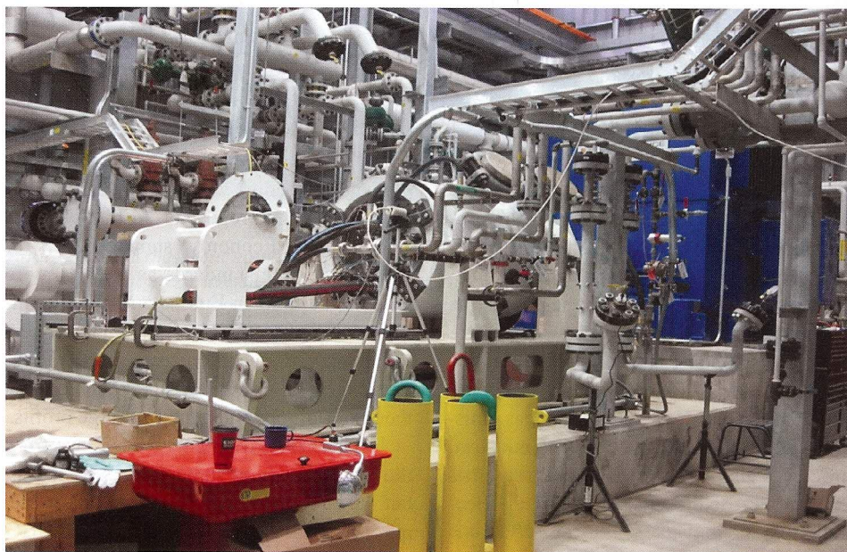
Figure 1 - Ramgen 8 MW, 10:1 pressure ratio CO 2 compressor being assembled for test on the Dresser-Rand dedicated closed-loop CO 2 test facility in Olean, NY, USA
